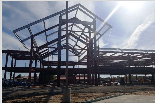
LEFT: Progress photo of the outdoor dining area trellis for the North County Campus Center cafeteria.
